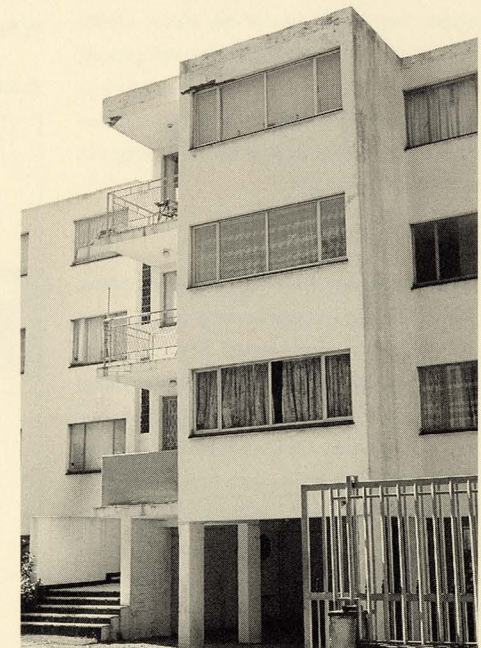
Example of International Style building (block of flats in Durban) showing cracking plaster.
